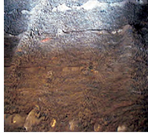
Steel screen mat shows 100% caking.
