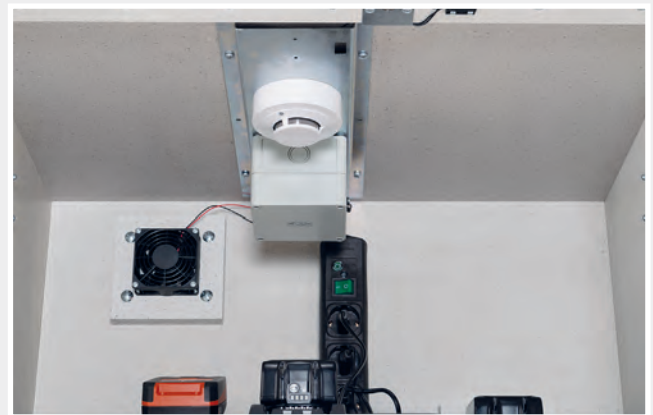
Battery charging cabinet from inside
